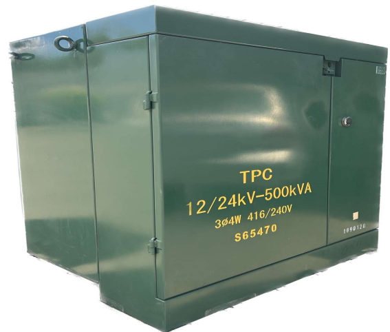
3Φ Pad Mounted Transformer
